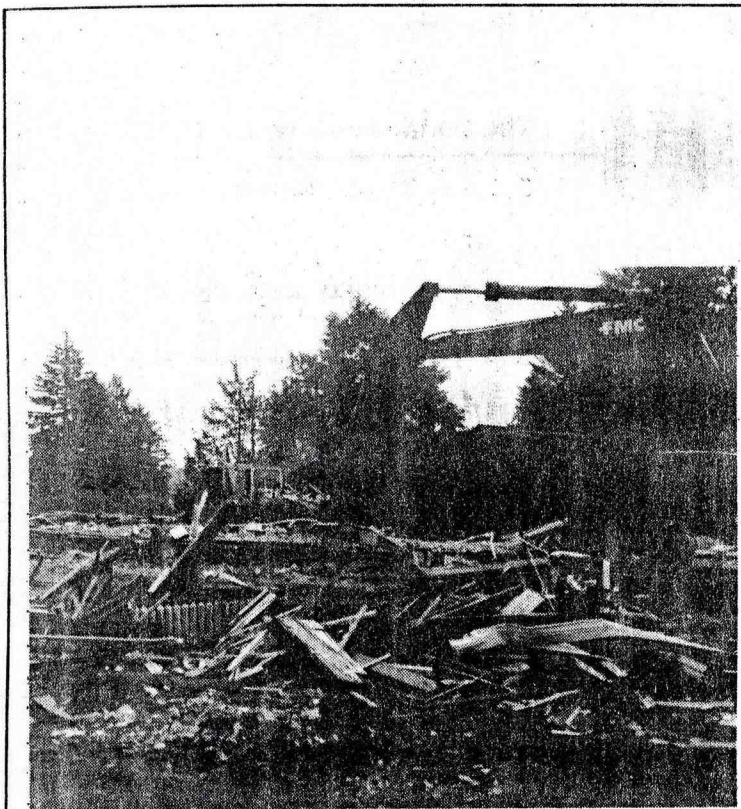
Down with the old and up with the new. Pictured here is the house beside the St. Mary's Church in West Lorne being demolished to make way for the new parish hall to be constructed.
